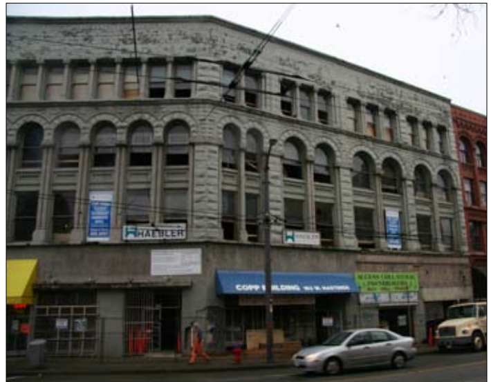
Pre-restoration. Note the loss of details
