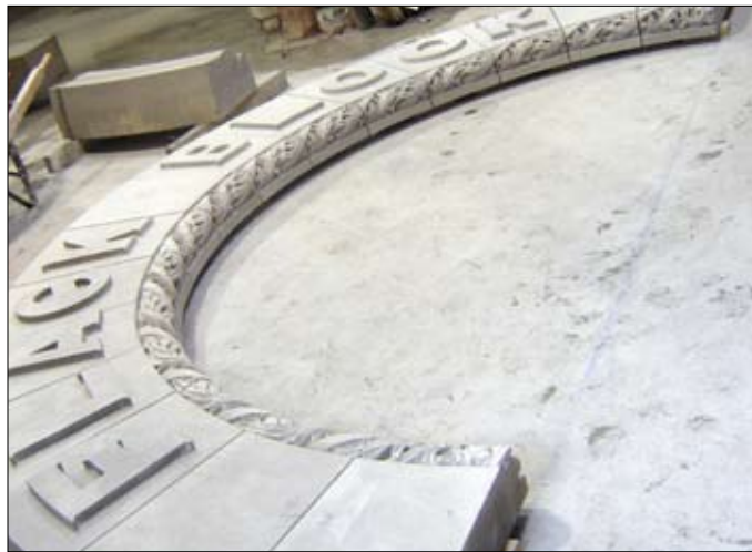
The new archway, in process and built in sections, yet to be installed
